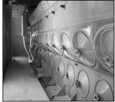
Interior view of a peaking plant generator.
