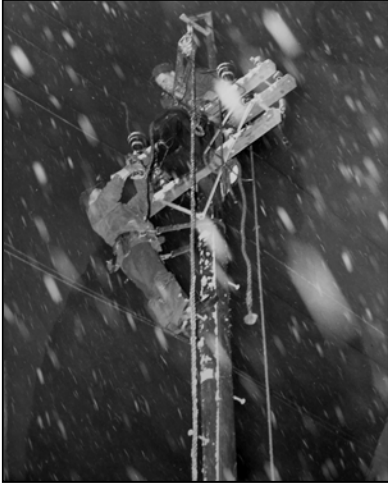
Shrewsbury linemen “Red” Rossboro [top] and Joe LeCoure repair damaged wires during a 1943 blizzard.
