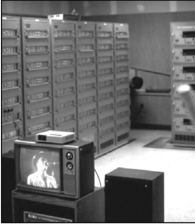
Shrewsbury Community Cablevision's Parker Road headend facility in 1983.
